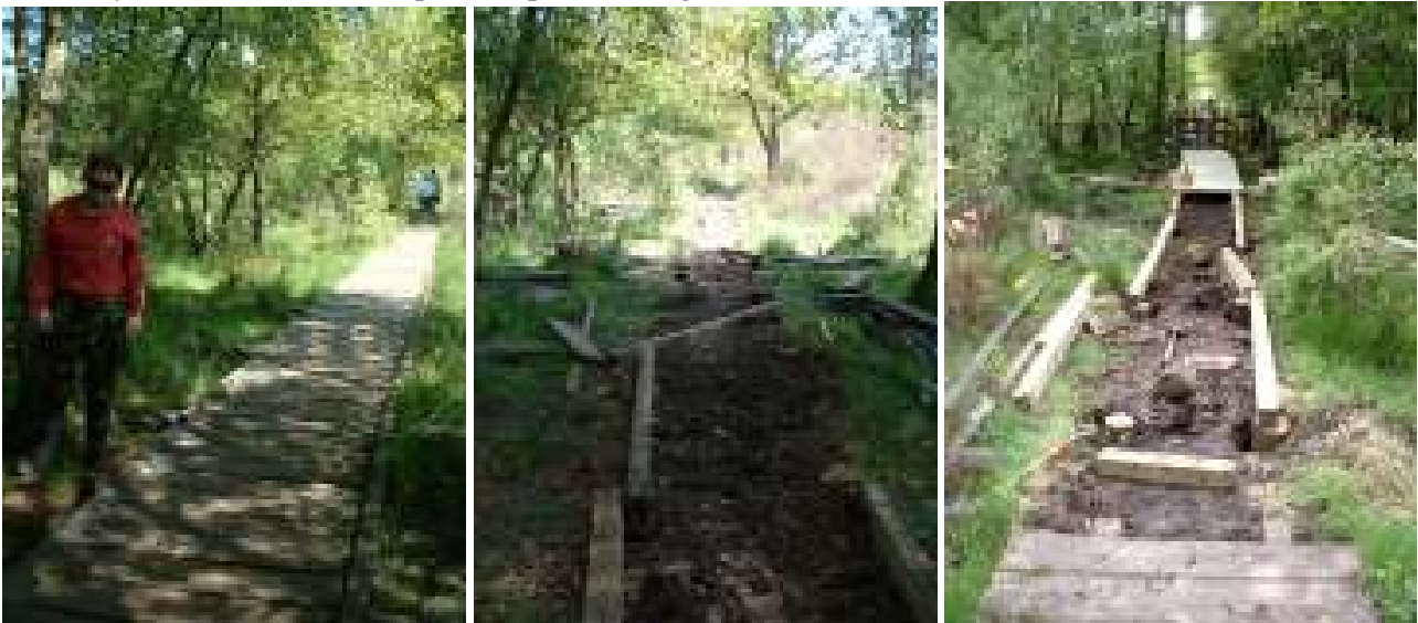
Above left – Phil inspecting the existing boardwalk. Above middle & right – Work in progress.
