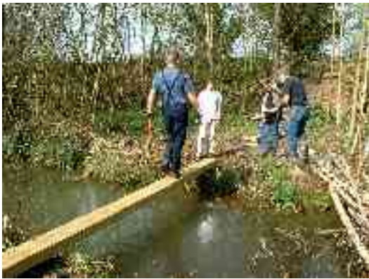
Above – Alisdair crosses the first plank as David, Nigel & Richard prepare the foundations for the bridge
