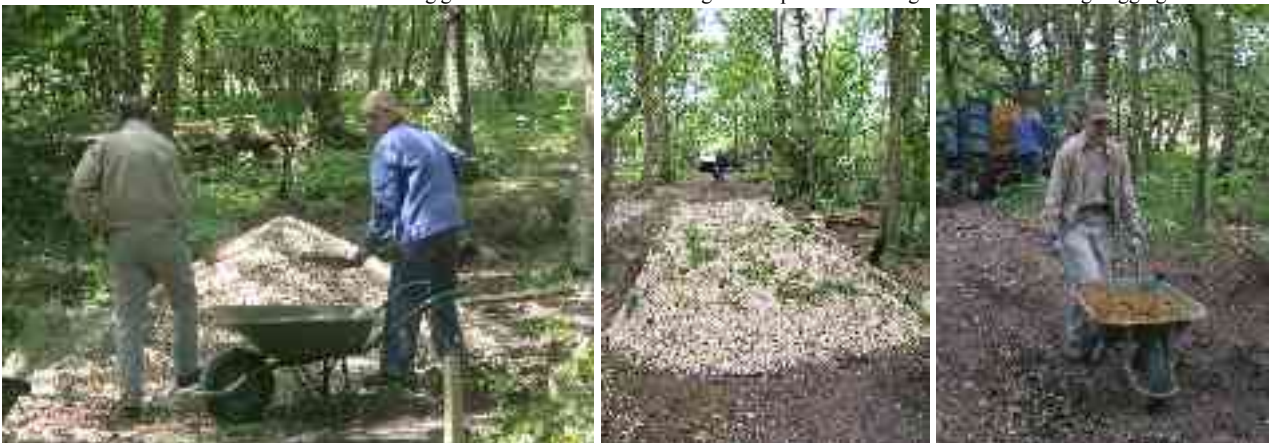
Below left – Peter & Anna shovelling gravel. Below middle – all the gravel in place. Below right – Peter barrowing hogging.
