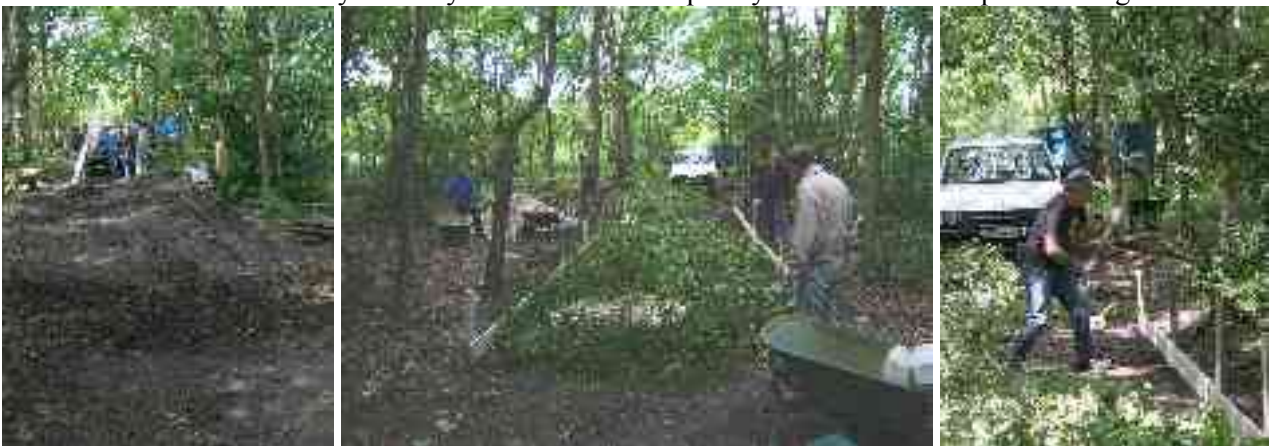
Above left – before. Above middle – the base layer of brushings. Above right – Richard knocking in a stake.
